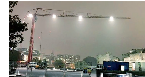
Four floodlights are mounted in the jib and tower.
